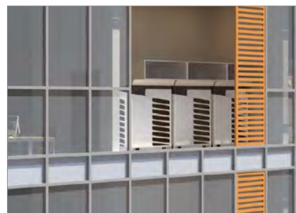
The outdoor unit is hidden inside the building without affecting the overall image of the building
